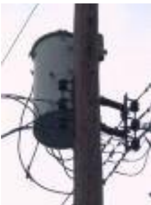
Transformers on poles.
