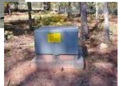
Transformers for underground power.
